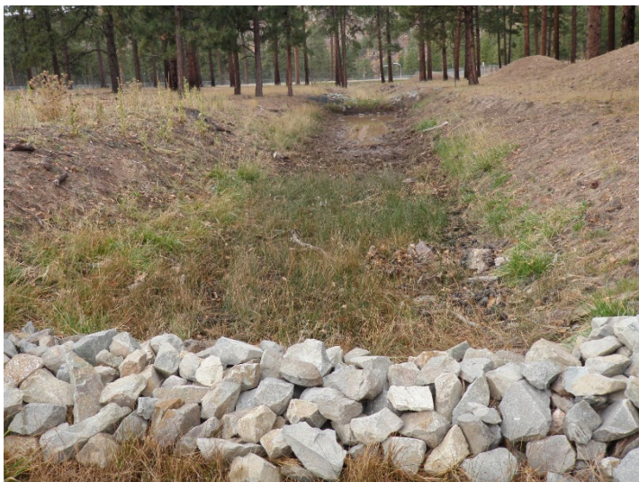
Sediment basin at W-SMA-1.5
