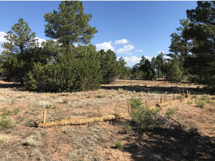
New stormwater controls at W-SMA-11.7
