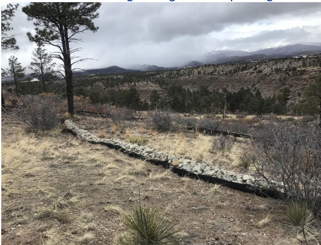
New stormwater controls at M-SMA-12.9
