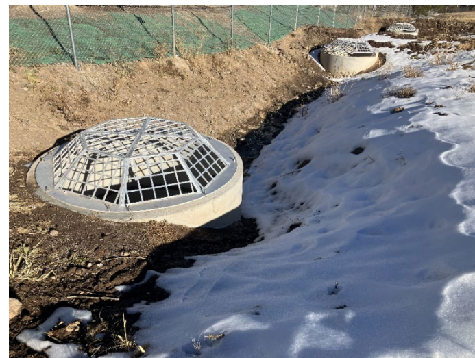
New stormwater controls at T-SMA-1
